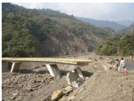
Photo 15 A bridge whose pier is only broken
