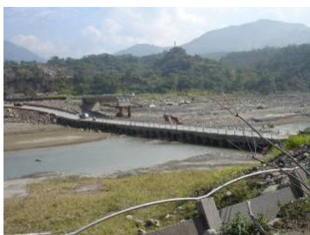
Photo 17 Buckling of steel pipe pile pier
