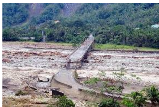
Photo 16 A bridge with broken abutment
