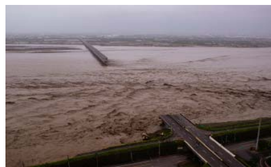
Photo 18 A bridge broken by local scouring
