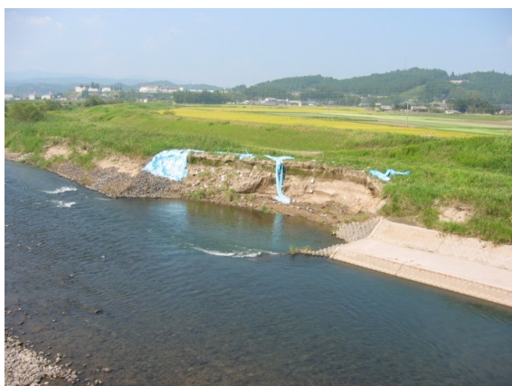
Fig. 7 Eroded river bank
