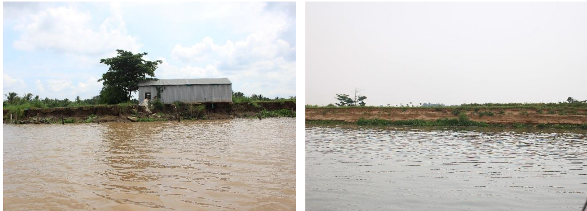
Figure 2.12 Typical river bank erosion in the Tien River. Photos were taken by Binh, D.V. during the field trip in August 2017.
