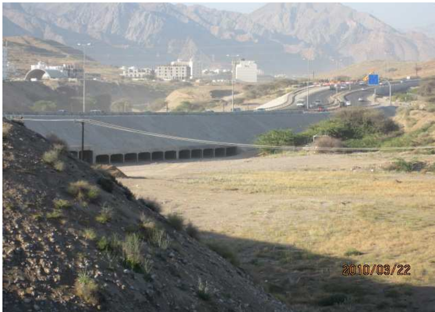
Figure 7.2 A box culverts constructed under a highway in Muscat City.
