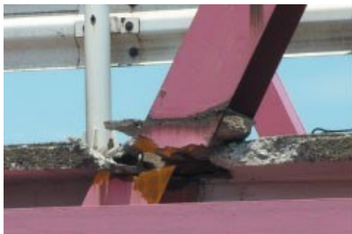
Figure 1.1 Photographs of the ruptured member on Kisogawa Bridge [2]
