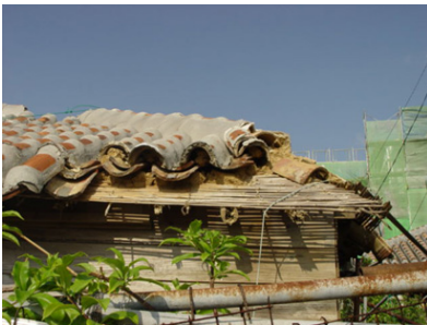
a. Damage to roof tiles.
