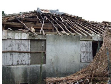
b. Blown off roof.
