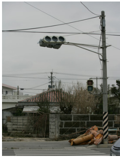
Photo 18 Distorted traffic signal. (Ishigaki city office presents)
