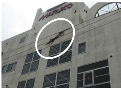
b. Damage to the wall.
