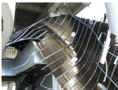
a. Fall down of ceiling panel.
