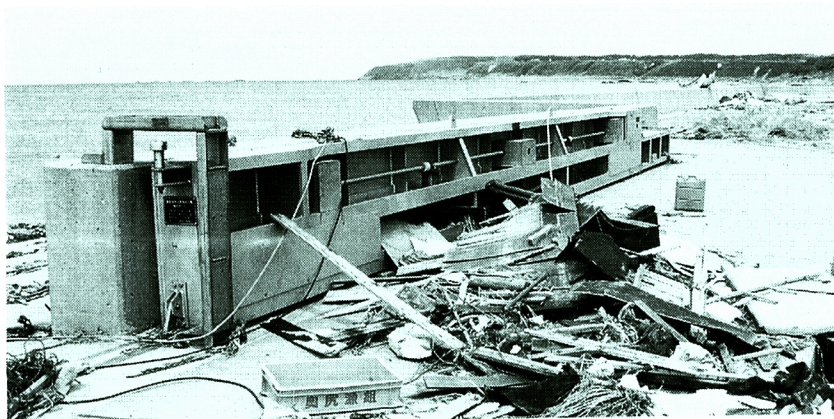
(a) Broken coastal dike
