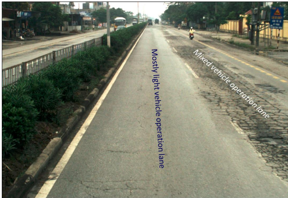
Figure 6.12 Typical pavement distresses on traffic lanes
