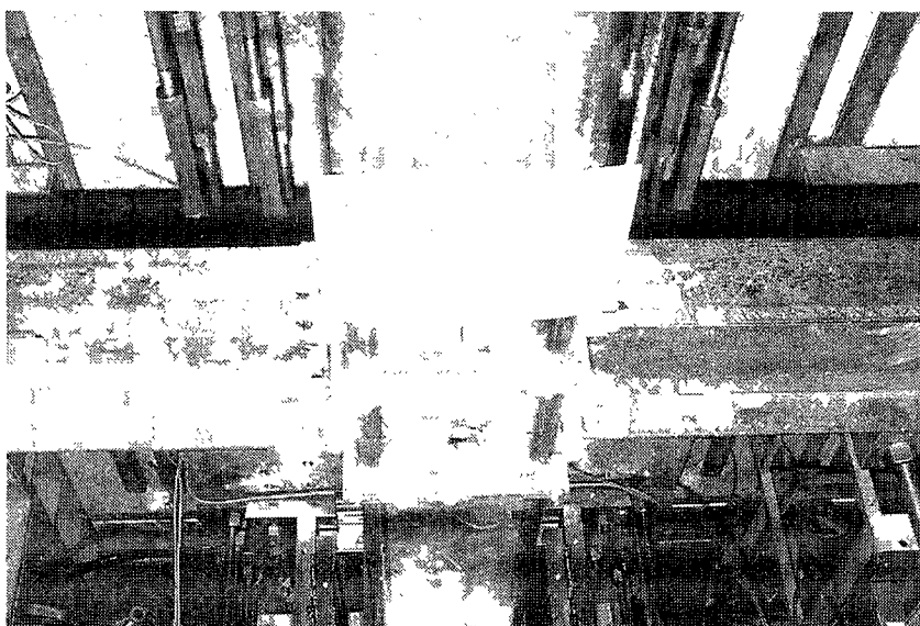
Photo 4 Fractured connection (conventional type)
