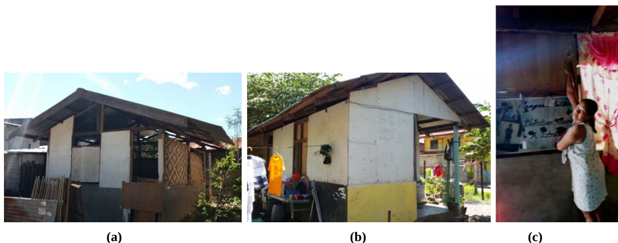
Figure 4.12: (a) Typical house built by PRC. (b) Damaged house repaired with improvised materials. (c) Level of water during Typhoon Bopha in Dec. 2012
