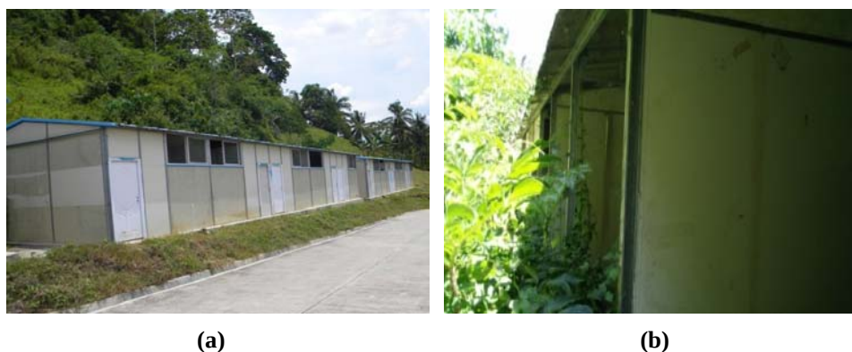
Figure 4.18 (a) and (b): Fifteen abandoned houses built by FCCC in a landslide-prone area
