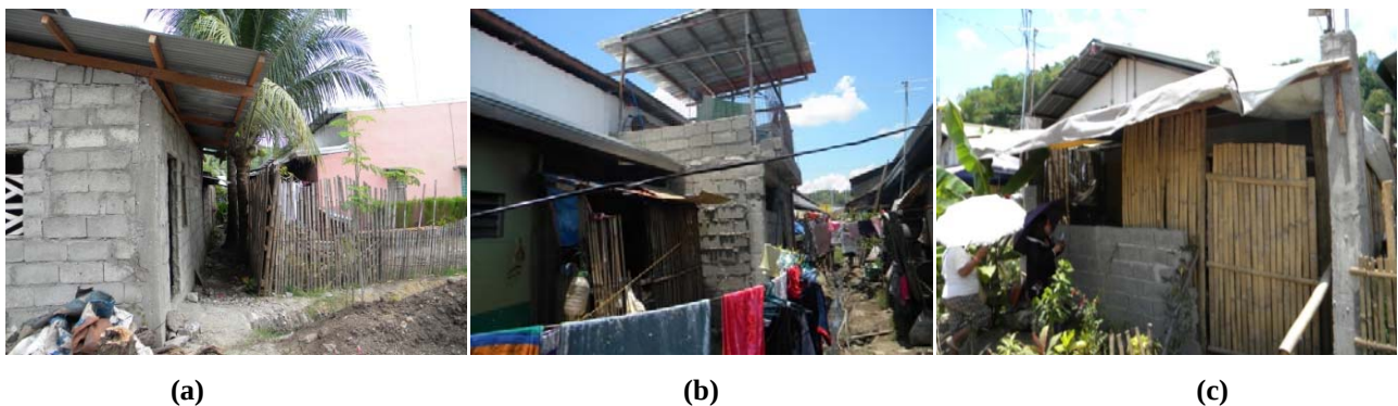
Figure 8.9: Roofing, wooden rafters and corrugated iron sheets (a), weak support of roofs (b), and improvised materials (c)
