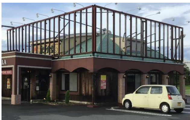
(a) 食堂看板の飛散
