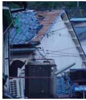
b. Damage to roof tiles
