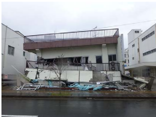
Photo 42 Totally collapsed building in Oroshimachi area
