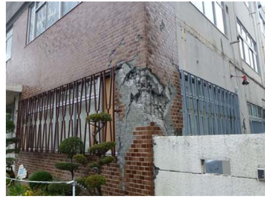
Photo 43 RC column damage in Oroshimachi area
