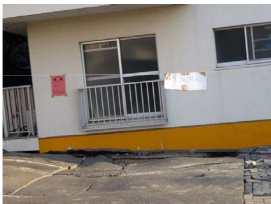
Photo 36 Totally collapsed building in Furukawa area
