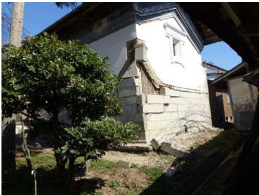
Photo 13 Damage of a storage in Shiwahime area
