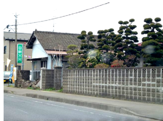
Photo 39 Damage of the concrete block wall
