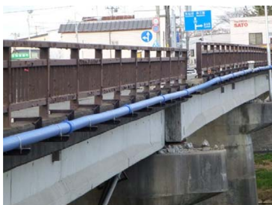
Photo 7 Displacement of Nishiki-bashi
