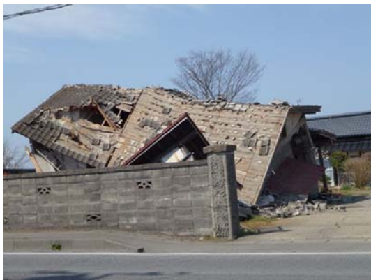
Photo 32 Totally collapsed house in Hirabari area
