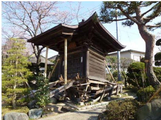
Photo 65 Damage of the building in Zuisen-ji
