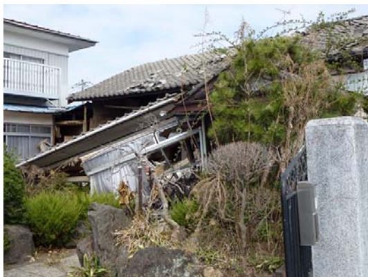
Photo 31 Totally collapsed house in Tajiri area
