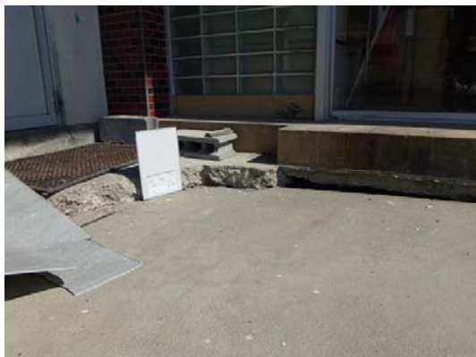
Photo 50 Damage of the foundation (site g)
