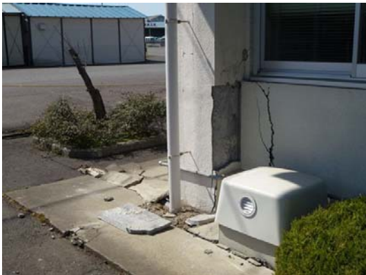
Photo 12 Seismic station at Shiwahime branch office
