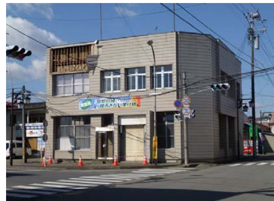
Photo 54 Damage of the exterior panel (site k)
