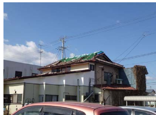
Photo 55 Damage of the roof tiles (site l)
