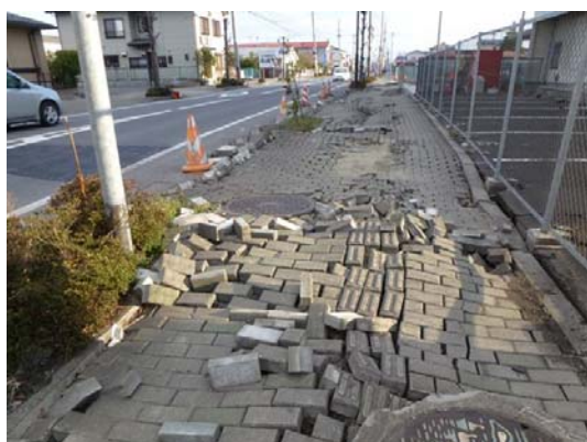
Photo 6 Ground damage in Sanuma area
