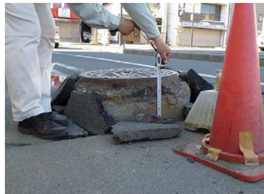
Photo 16 Floating of a manhole in Wakayanagi area
