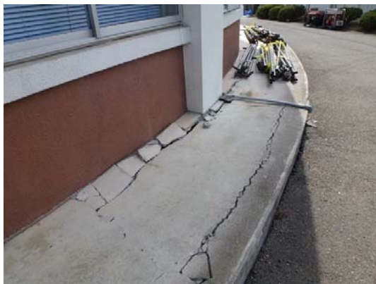
Photo 30 Base damage of the Tajiri branch office
