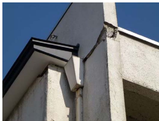
Photo 3 Building damage of Semine branch office
