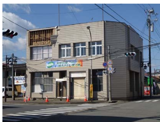
Photo 10 Damage of the wall in Tsukidate area
