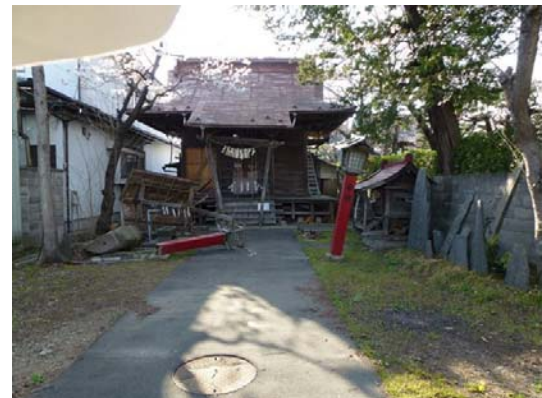
Photo 70 Damage of Nishinomiya shrine on 4/18
