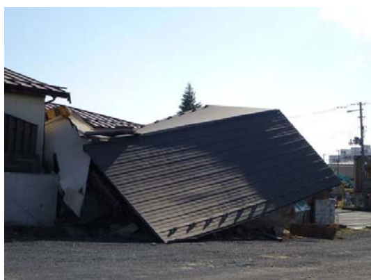
Photo 5 Totally collapsed house in Sanuma area
