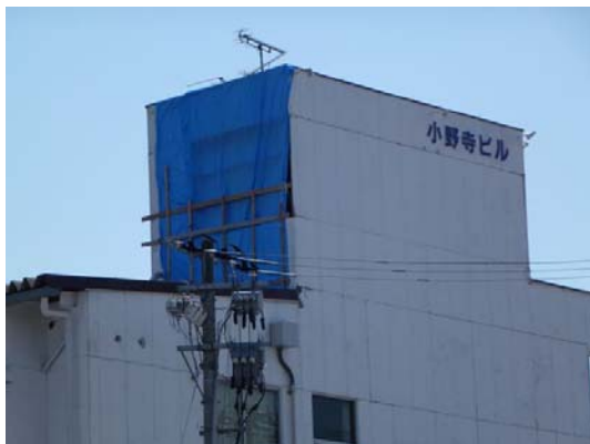
Photo 49 Damage of the exterior panel (site f)
