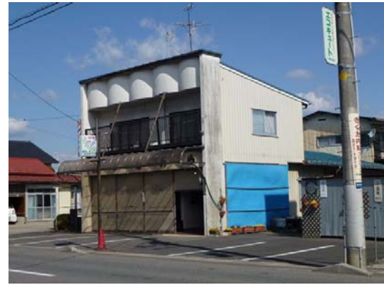
Photo 52 Damage of the exterior wall (site i)
