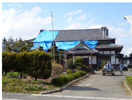
Photo 4 Damage of the roof tiles in Naganuma area
