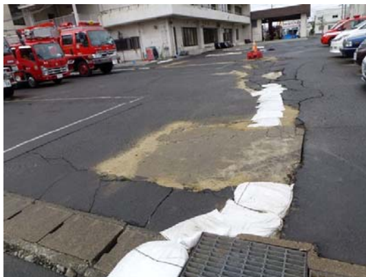
Photo 41 Ground damage at Miyagino fire station
