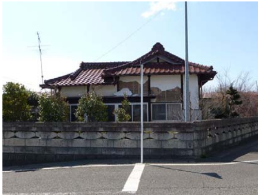
Photo 48 Damage of the plaster wall (site e)
