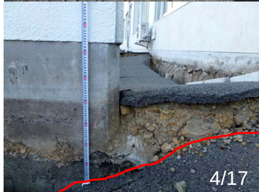
Photo 62 Comparison of the damage of ground pavement
