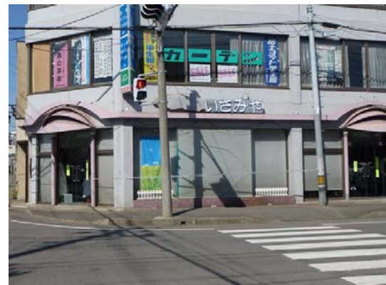
Photo 53 Damage of the glass window (site j)
