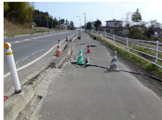
Photo 27 Ground damage along the prefecture route 1
