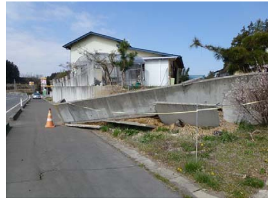
Photo 26 Ground damage along the prefecture route 1
