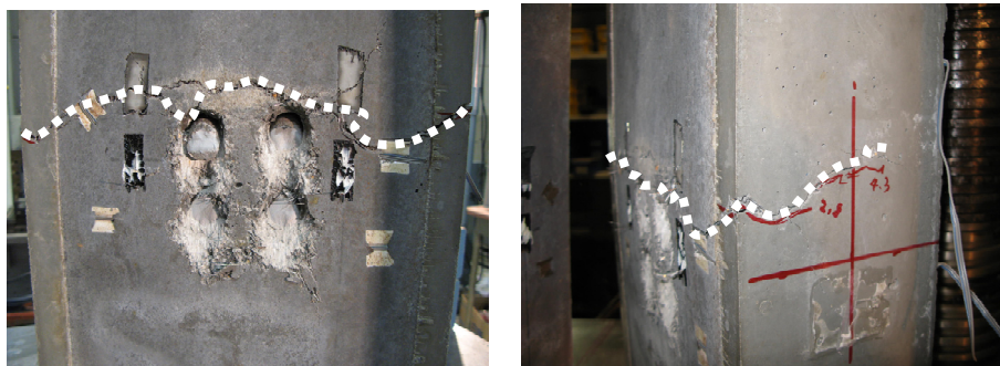
Fig. 5. 13 Transverse crack in Specimen ‘4PG50’
