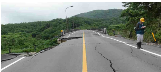
(a) damage of girder: center line inclined
