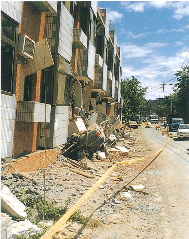
Collapse of the 1st floor in a 3 story building located in Chungliao. (Photo3)
