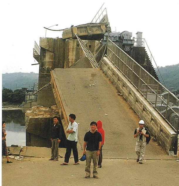
Road along the top of a dam that is vertically offset by fault. (Photo2)
