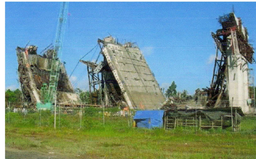
Fig.14 Collapsed concrete girder
