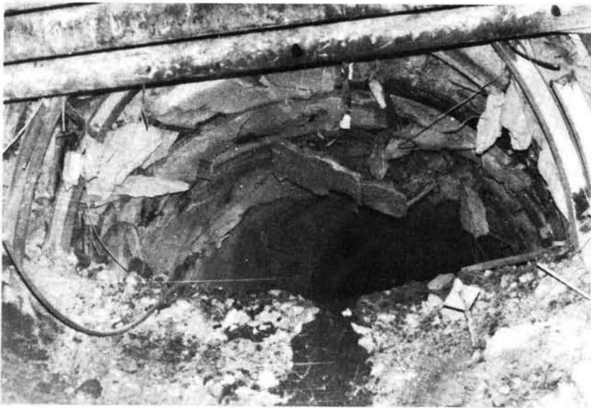
Photo 10.3 Observed Collapse at STA. 33 km 225 m – 255 m
