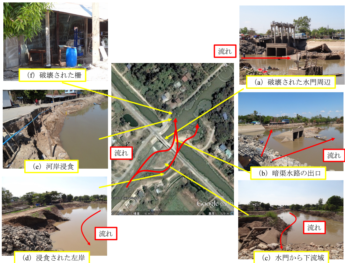
Fig. 6 Erosion around the gate at Bang Chom Sri.
