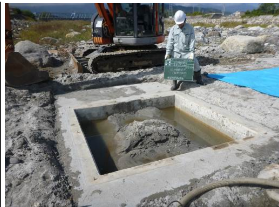
Photo 1: Sedimentation in the pit (2014 Typhoon No. 18)
