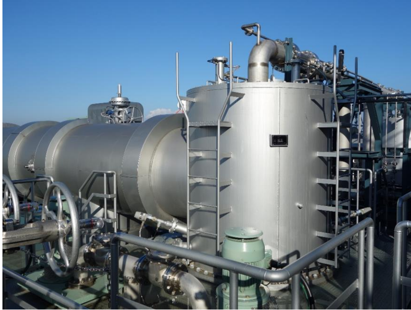
Figure 2.6 Photograph of large-scale SCV burner.
