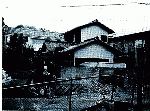
Photo 1 Earthquake damaged House SU (Nishinomiya).
