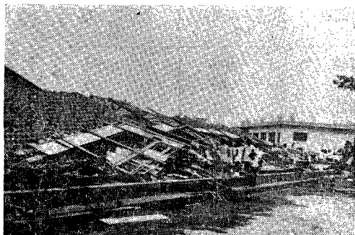
Photo. 2 Collapse of a wooden school-building.
