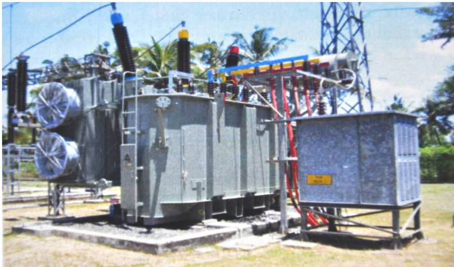
Figure 2.4 The power transformer
