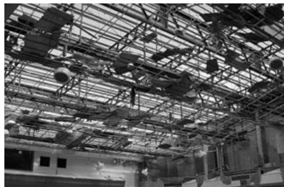
Photo 6. Blow off of a gymnasium roof.
