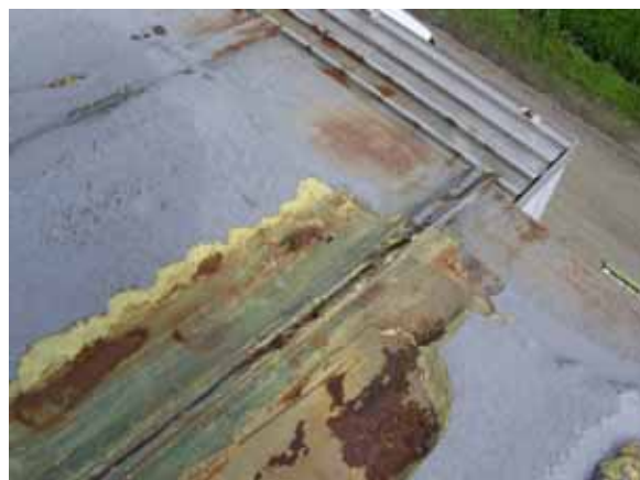
Photo 7 Remained roof surface.
