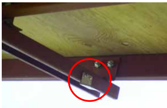
Photo 8 Blown roof and shackle
