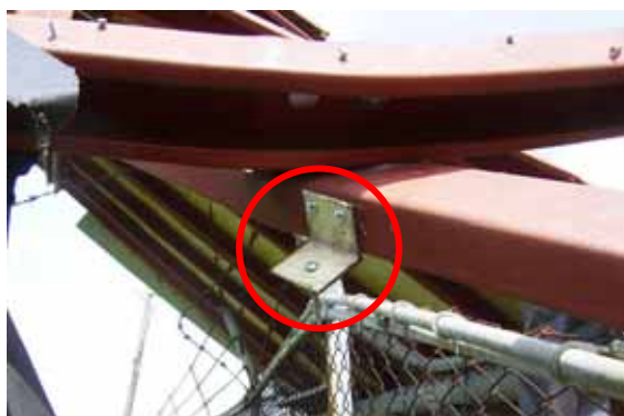
Photo 9 Blown roof and shackle
