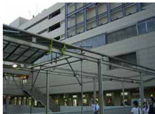
Photo 3 Blown away roofs on a pedestrian bridge.
