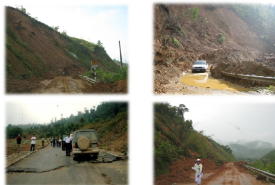
Landslide along Ho Chi Minh National Highway
