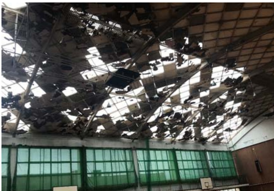
Fig.22 damaged roof of gymnasium (科研費報告書, 2019)
