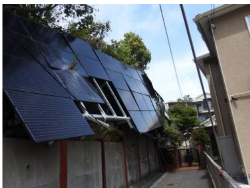
Fig.33 damage to solar panels (科研費報告書, 2019)
