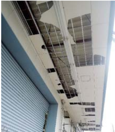
Fig.27 damage to building eaves (科研費報告書, 2019)
