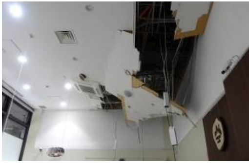
Fig.26 damage to the ceiling (科研費報告書, 2019)
