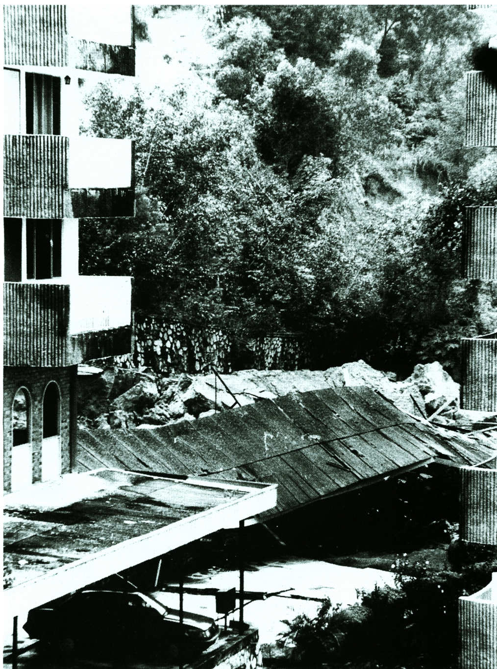
Photo 1 Starting landslide behind the building.
