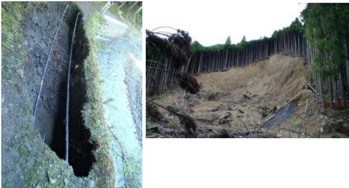
Figure 4.2 Severely damaged part of the Nakahechi Route due to flooding (left) and landsliding (right). Photos were taken by the author in 2013.
