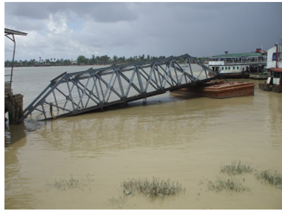
Photo 4 Damage of connection bridge
