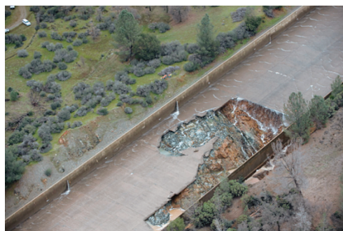
Fig. 2 Oroville dam spillways incident (Matsumoto, 2017)
