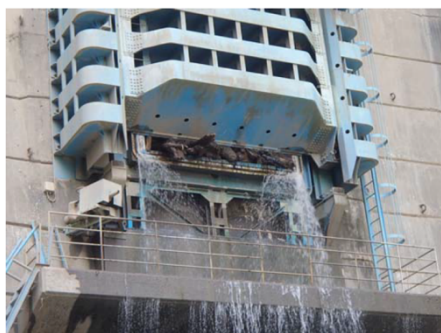
Fig. 1 clogging of outlet of Susobana dam (MLIT, 2018)
