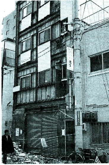
Photo 22 Steel structure with loss of cladding.
