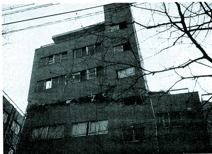
Photo 17 Collapse of upper stories.
