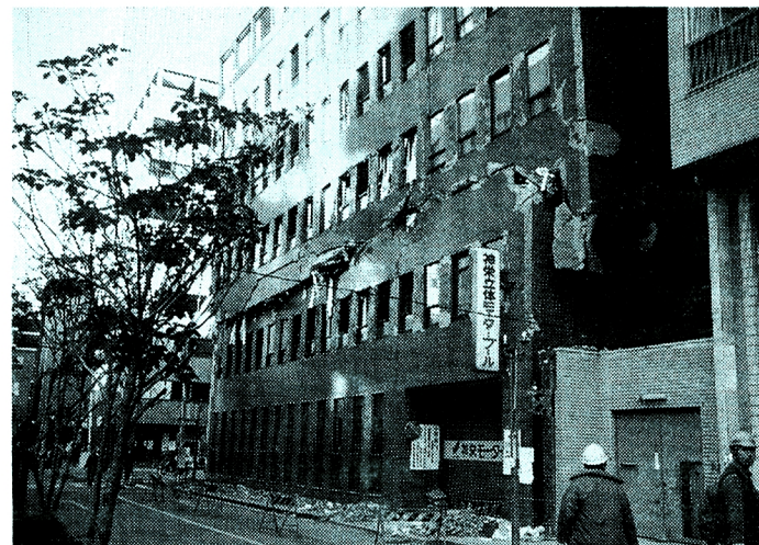
Photo 14 7-story building with a collapsed 3rd story.
