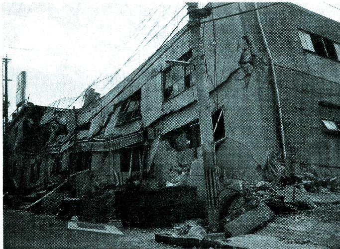
Photo 19 Collapse of a factory building.
