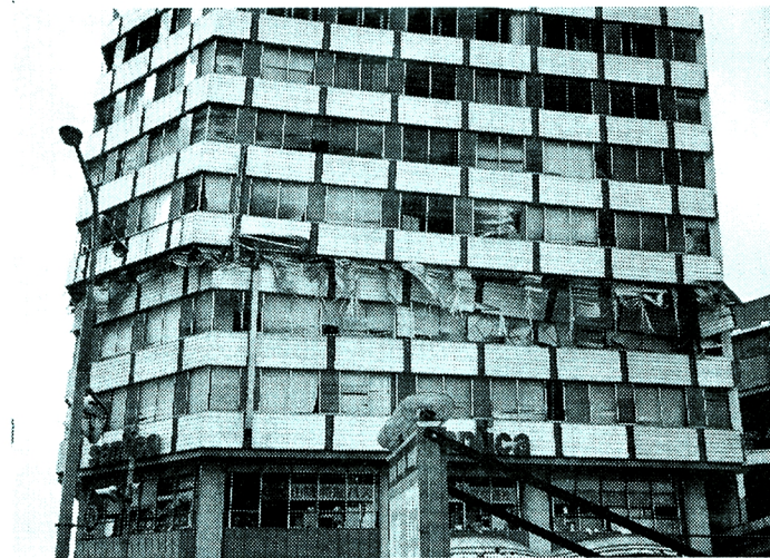
Photo 13 9-story building with a collapsed 5th story.
