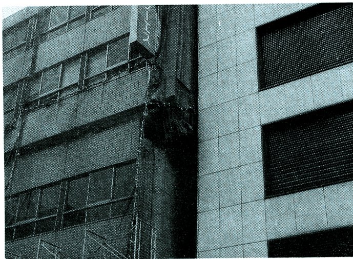
Photo 15 6-story building with a collapsed 4th story.
