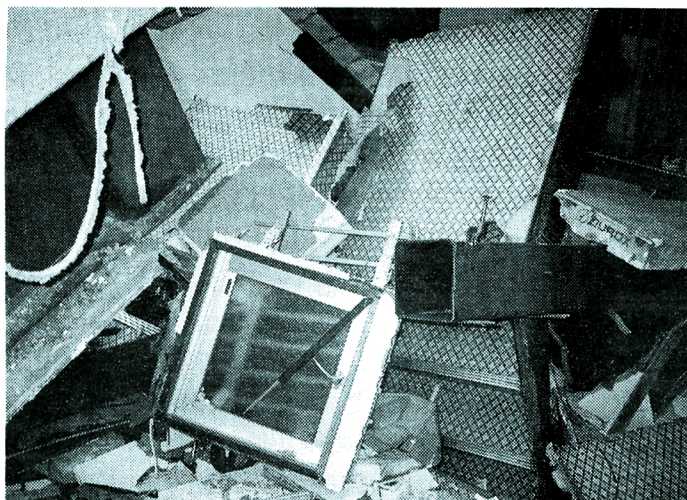
Photo 27 Failure at the top of column.
