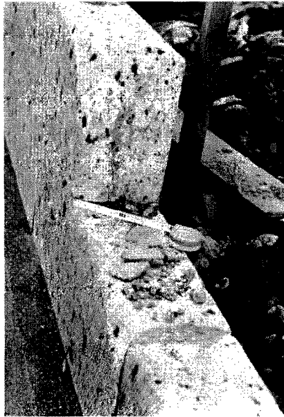
Photo. 8 Collapse of a block fence.
